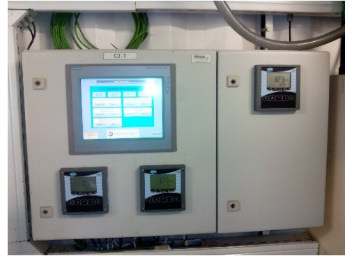
Figure 3.6: The pilot plant control interface - PLC.
